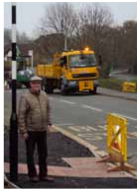
Brian in Ladybridge Drive as the work progresses on the pedestrian crossing.
